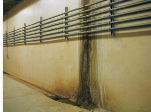
Leaking crack in wall
