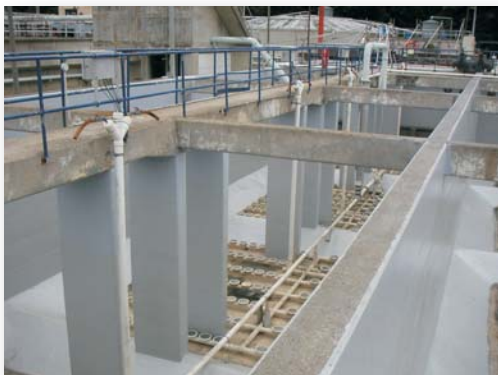
Completed aeration tanks
