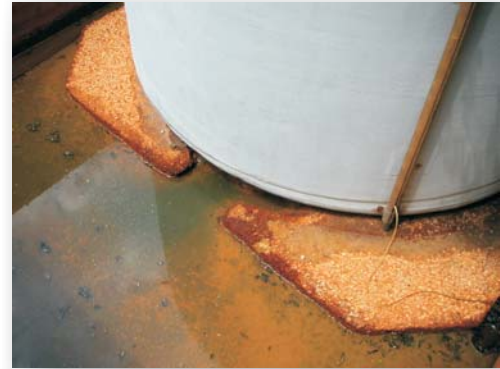
Old tank and deteriorated concrete pad
